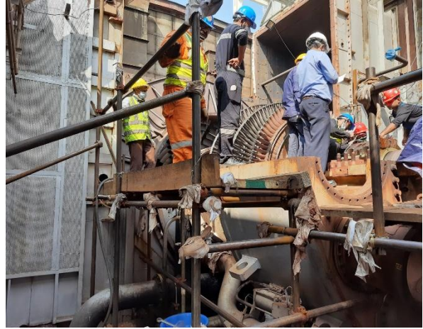
Maintenance in Power Plant
