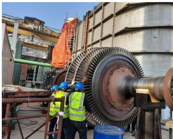
Maintenance in Power Plant
